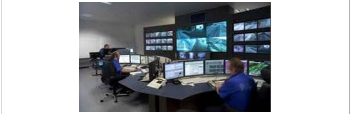
출처 : Advanced Traffic Signal Controller(City of Dallas)
