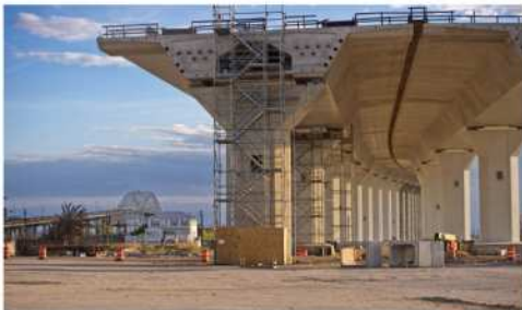
Construction on the northern portion of U.S. 181 leading to the Corpus Christi Harbor Bridge in Texas. Photographer: Eddie Seal/Bloomberg
