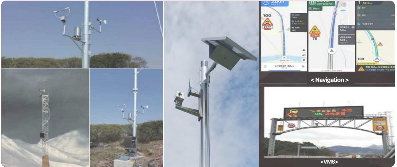
▲ Sensors mounted on highway CCTV poles monitor road weather hazards, such as black ice, and promptly relay the information to drivers.
