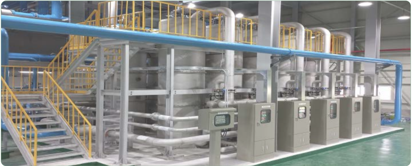
▲ The water treatment center at Kolon Industries' Gumi plant (14,400 tons/day) purifies water in just 3 minutes using fiber filtration systems.
