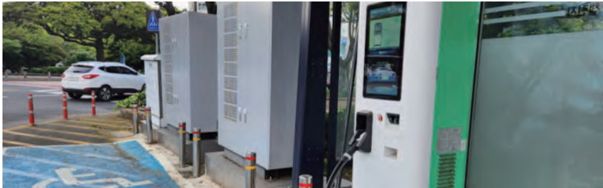
Electric Vehicle Charging Station
